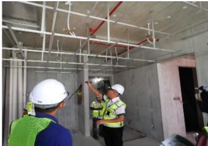
Figure 52: Post dismantlement of an aluminium formworks system at Serviced Residences Tower, BBCC
