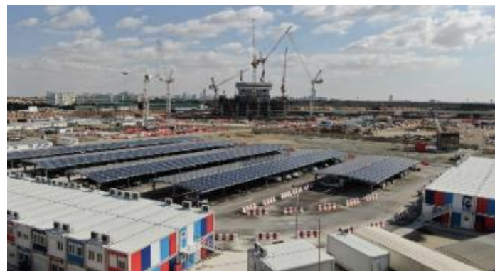
Figure 7: Carpark-mounted solar panels at Besix's 340m skyscraper construction site
