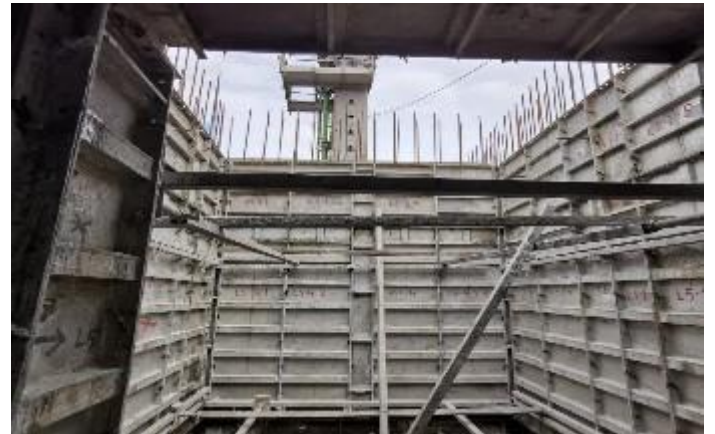
Figure 51: Aluminium formworks usage at Serviced Residences Tower at Bukit Bintang City Centre (BBCC) project
