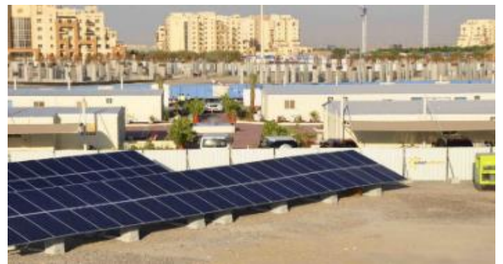
Figure 8: Solar panel at Remraam residential development project site
